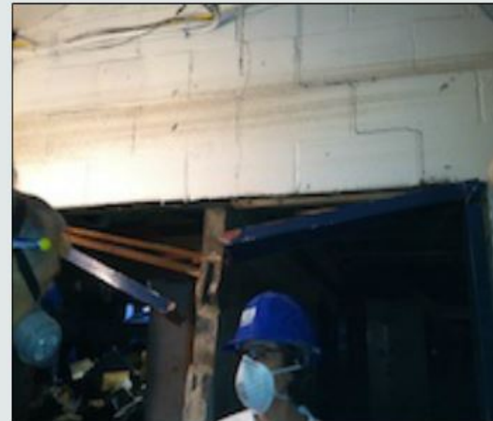
Structural Damages, Petroleum, Mold - Hurricane Sandy 20
